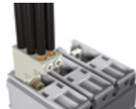
Multi-cable terminals with cables
