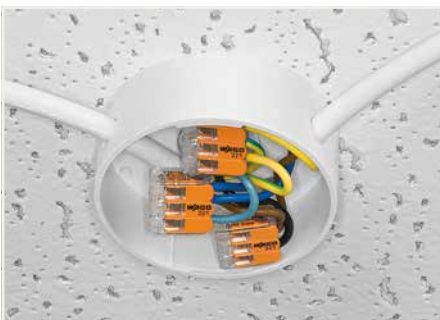
Lighting distribution in ceiling canopy
