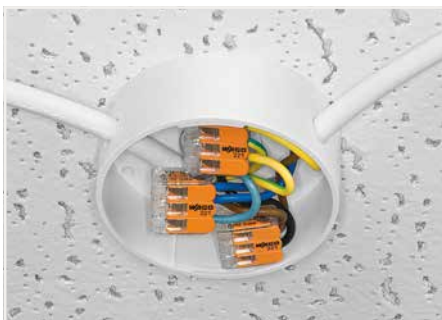
Lighting distribution in ceiling canopy
