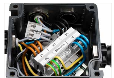
Wiring example in an Ex junction box
