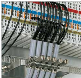
Installation on U-shaped copper busbar
